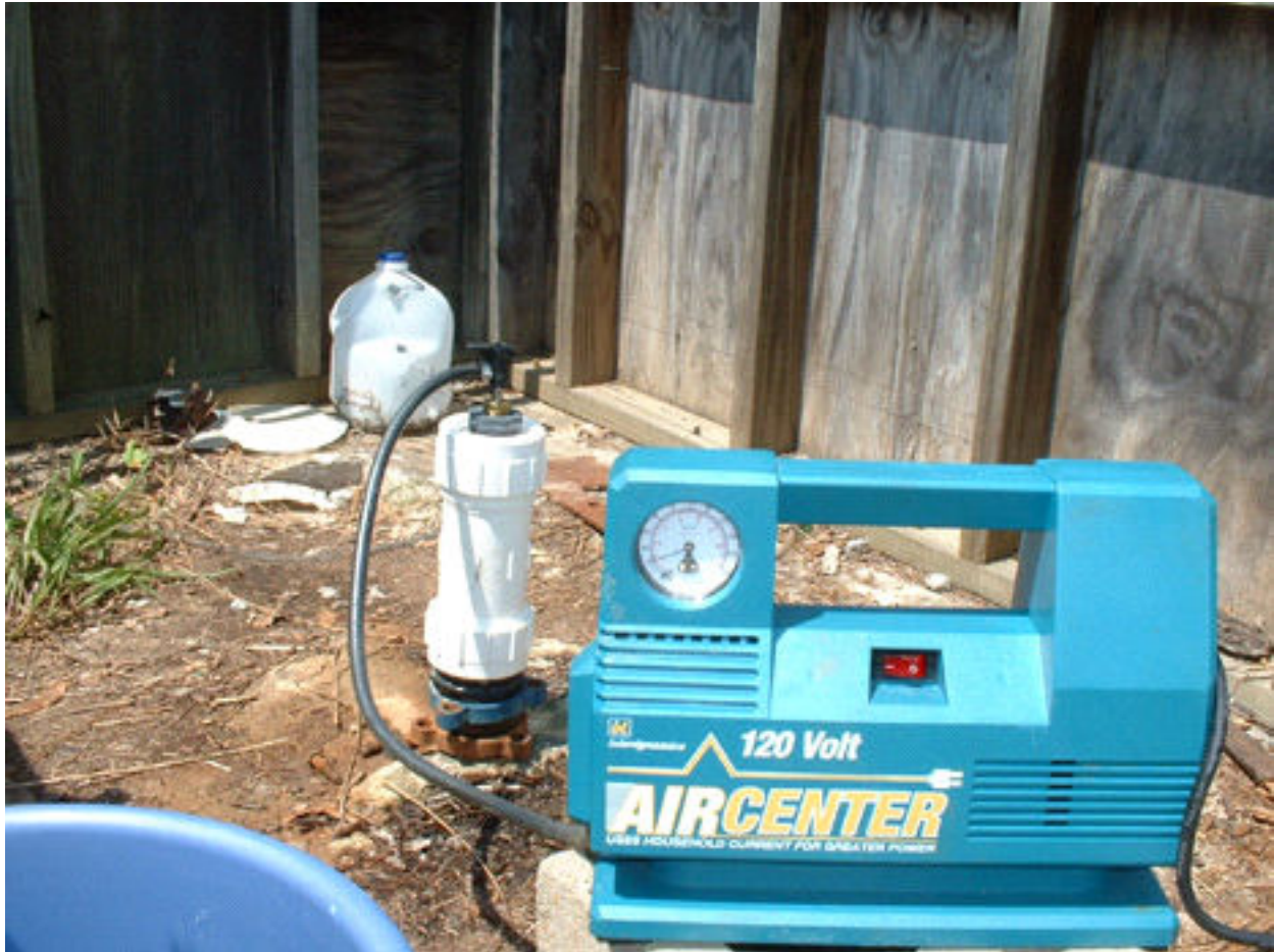
Figure 4.11. Air injection apparatus for solution displacement, well Bogey C
